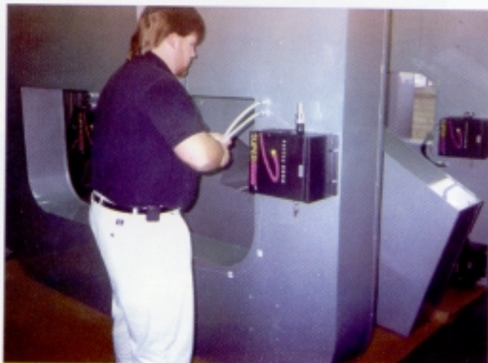
Fig. 3: The illuminator boxes containing 150-watt metal-halide lamps and color wheels are attached to the backs of the letters.
